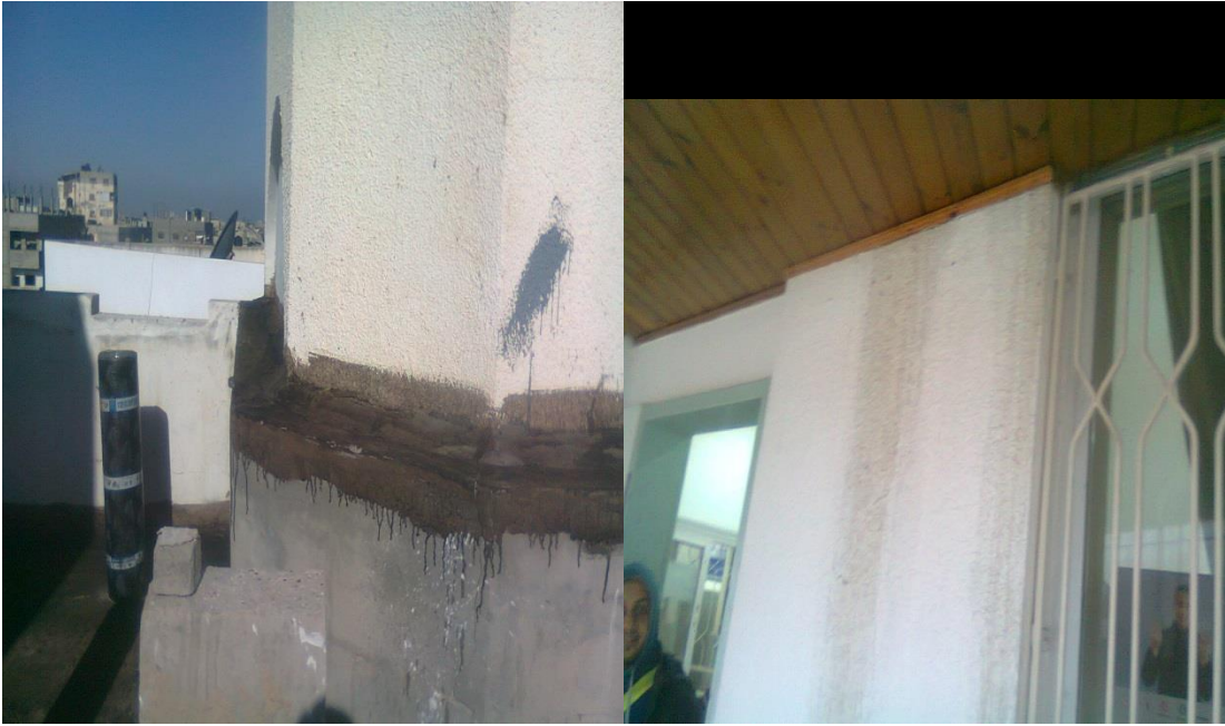
Figure 6.7: Water leakages through joints
