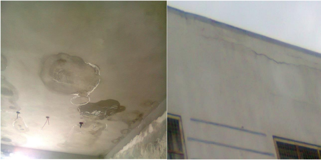
Figure 6.5: Staining of ceiling boards
