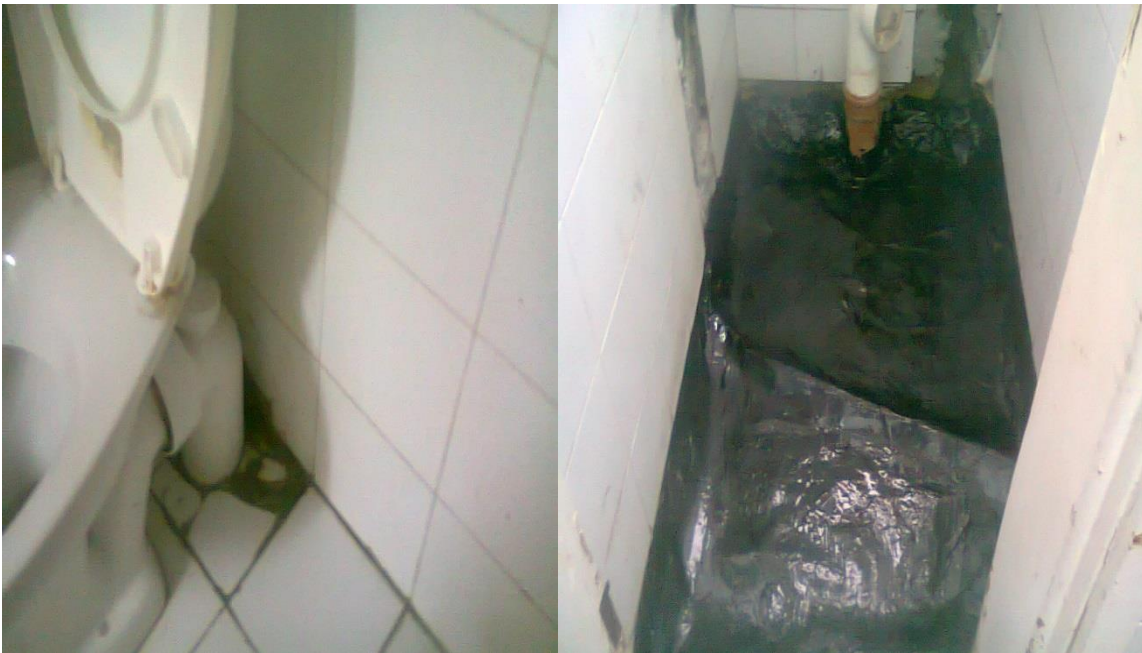
Figure 6.6: Water leakages through pipe penetration
