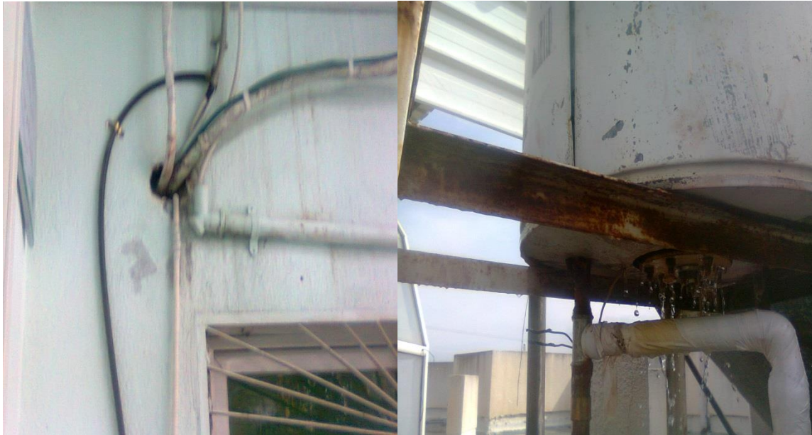
Figure 6.10: Corrosion of exposed drainage pipes
