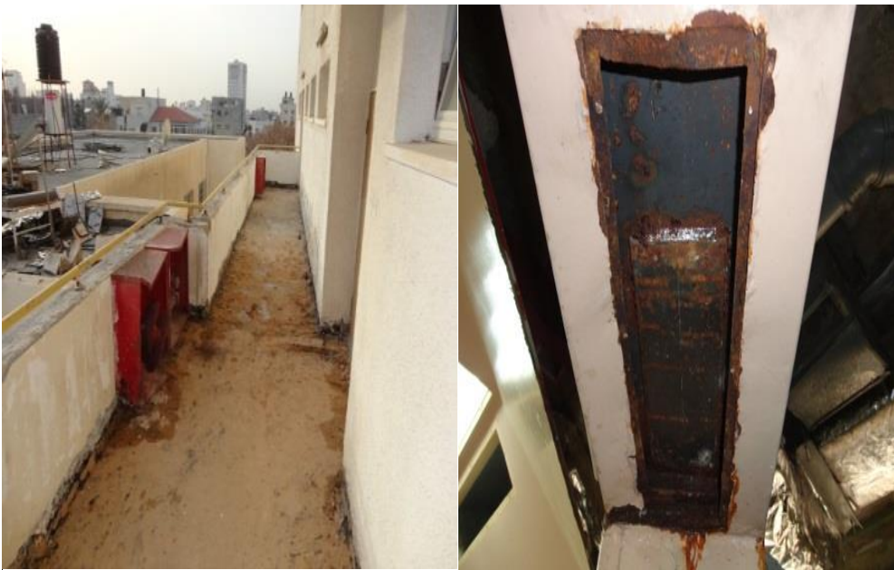
Figure 6.8: Corrosion of exposed drainage pipes
