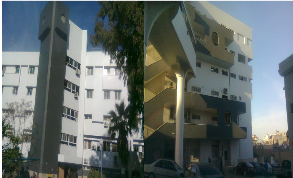
Figure 6.11: Corrosion of exposed drainage pipes
