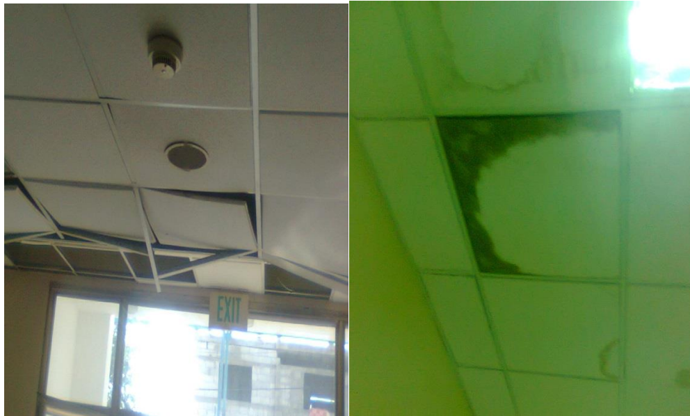
Figure 6.4: Staining of ceiling boards
